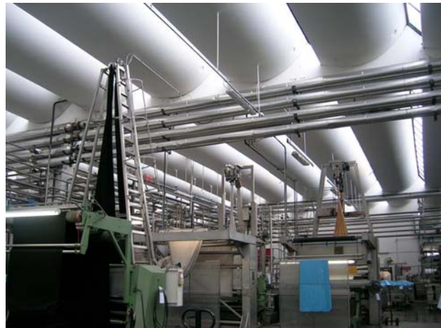
Inside of a finishing mill
